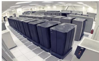
HPC Processing center
